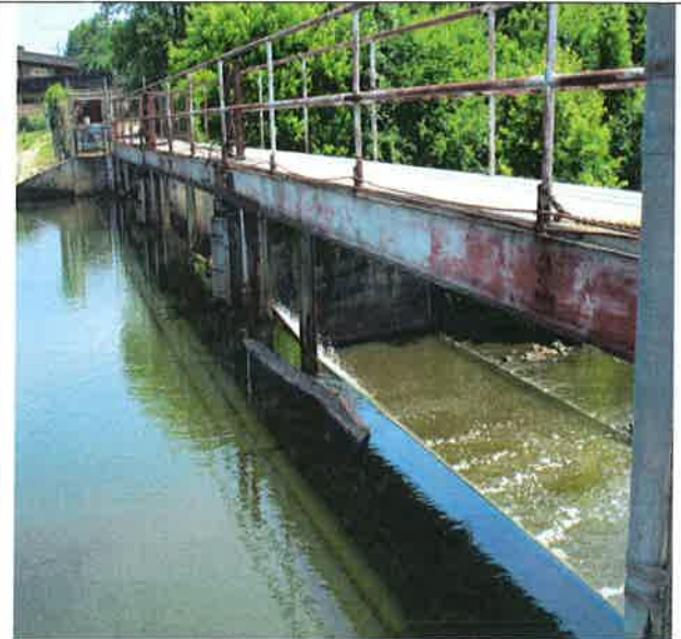
Log on Spillway
