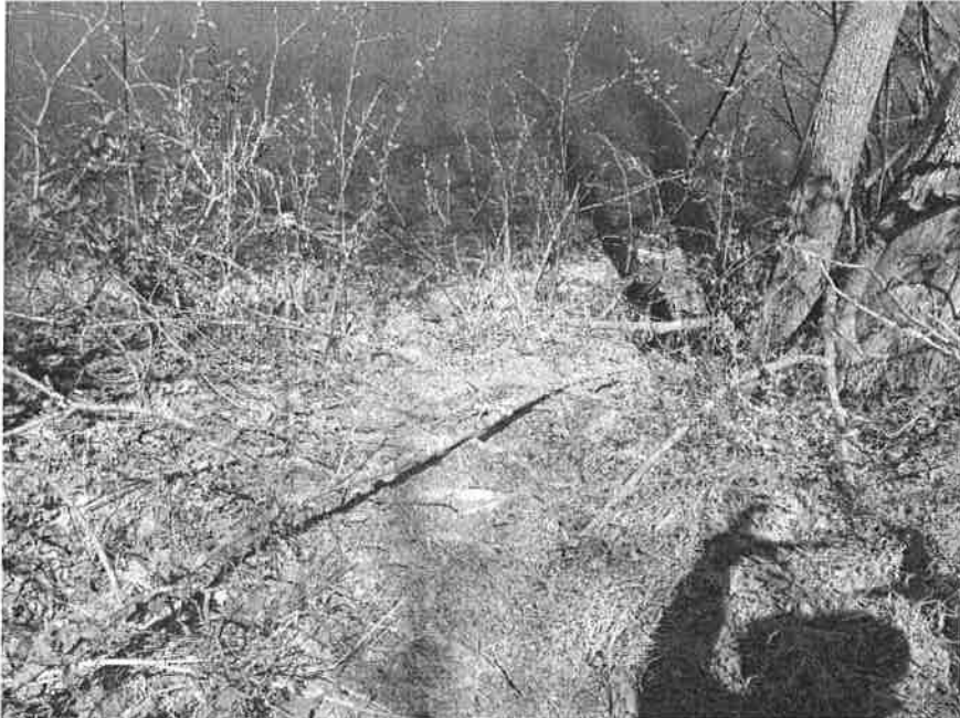
Sloughing present throughout the slopes on the dam
