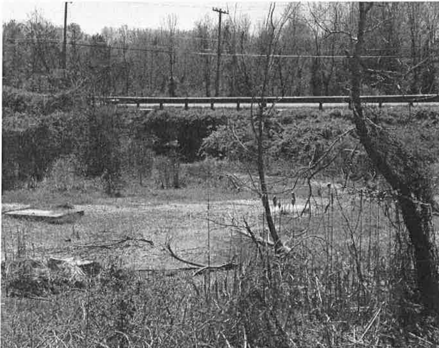
Evidence of sloughing on the downstream slope, sliding debris, seepage at the toe of the dam and the downstream this is causing standing water. Very close to highway, may flood in case of failure.
